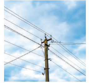
Electrical and Utility
